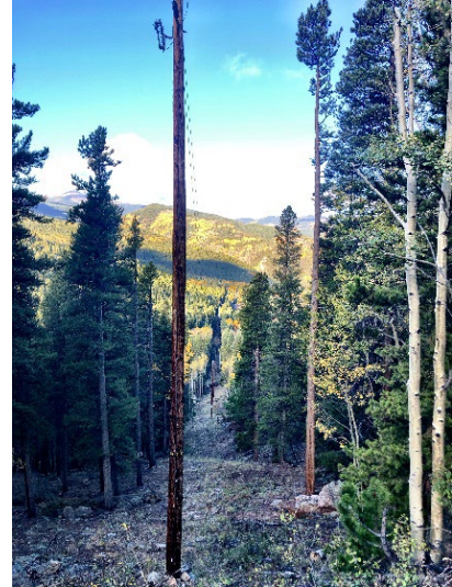
Company right-of-way with requisite clearances
